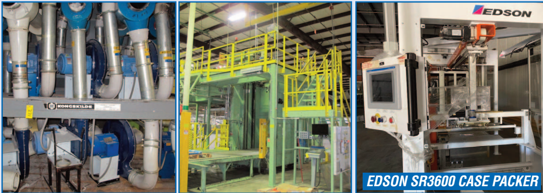
PARTIAL VIEW OF MOTORS, SERVO DRIVES, ELECTRICAL, MCC'S, TRANSFORMERS
